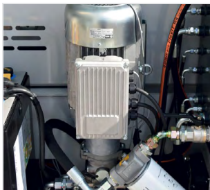
A/C electric power unit
