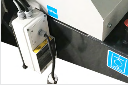
Thermal-magnetic switch panel and power line inlet.
